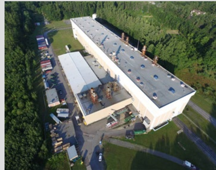
Saint-Gobain Performance Plastics Corporation – Merrimac, NH Currently installing a thermal oxidizer to treat exhaust
